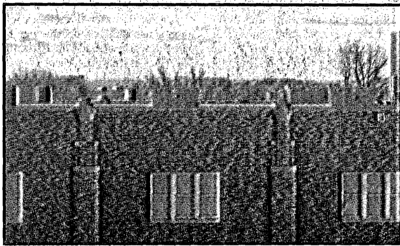
The new heating and cooling units on the roof of the City Auditorium are visible from the City building across the street.
